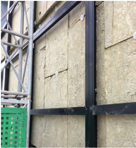
Insufficient fixings in insulation.
