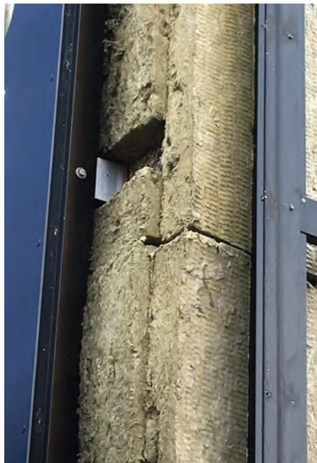
Gaps in insulation and support structure missing.
