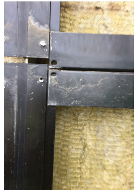
Missing support structure fixings.
