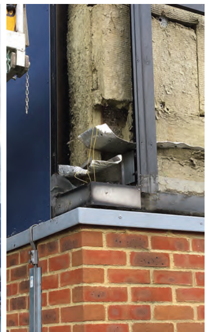
Incorrectly installed firebreaks and gaps in insulation.
