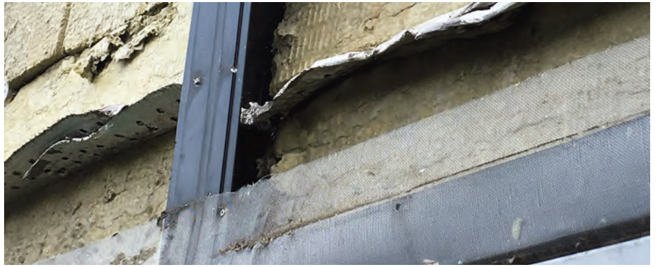
Incorrectly installed firebreaks.
